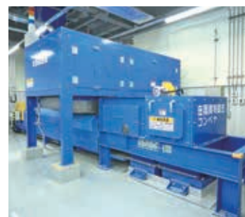
7 Conveyor for removal of foreign objects from cans
