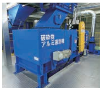
5 Aluminum sorting machine for crushed materials
