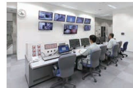
6 Central control room
