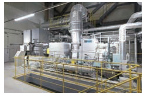
4 Steam turbine generator
